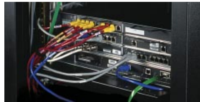
This Cisco 7200 Series router acts as the core gateway to Altera's corporate wide area network (WAN) and the Internet.
