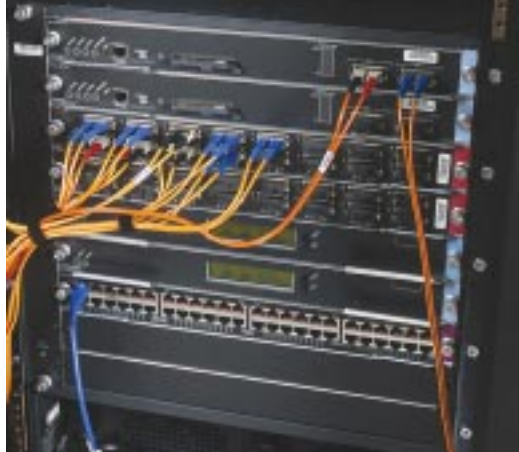
Switches from the Cisco Catalyst 6500 family, like this one, are at the heart of Altera's LANs.
