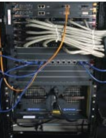
Altera's corporate network is almost entirely composed of Cisco routers, firewalls, and other products, like this Cisco Catalyst 5500 switch, which is used to support Altera's local area networks (LANs).
